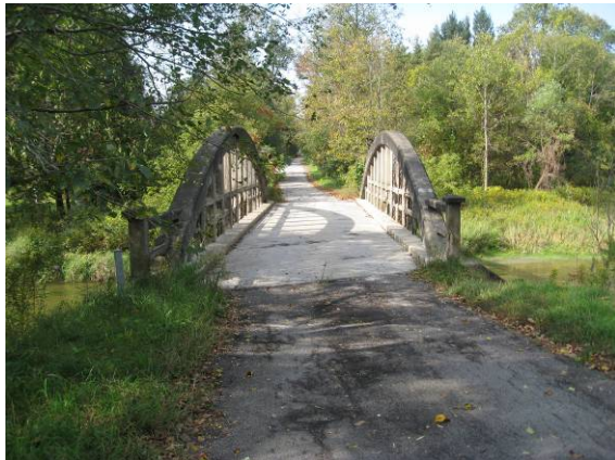
Plate 3: View southwest across bridge. Note flood plain on both sides adjacent to river.
