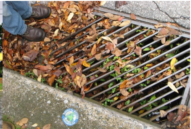
Partially blocked curb/gutter drain reducing stormwater capture efficiency
