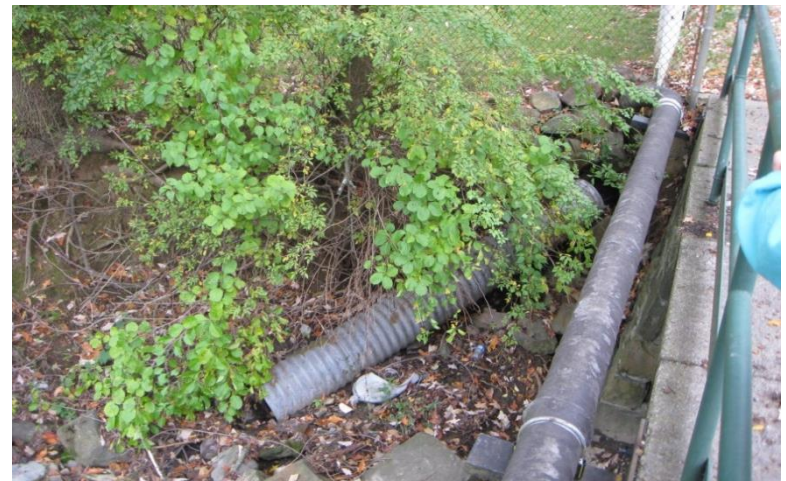
Erosion causing failure of a stormwater outfall
